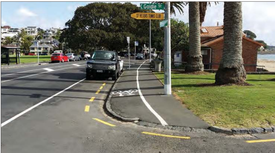
Figure 12.1: Substandard shared pathway next to parking, Auckland, New Zealand. (Source: Author.)
